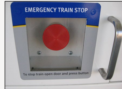
Platform Emergency Stop Button
