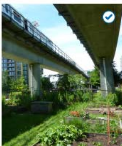
A community garden demonstrates positive use of residual land under elevated trackway. Joyce-Collingwood Station, Vancouver, BC.
