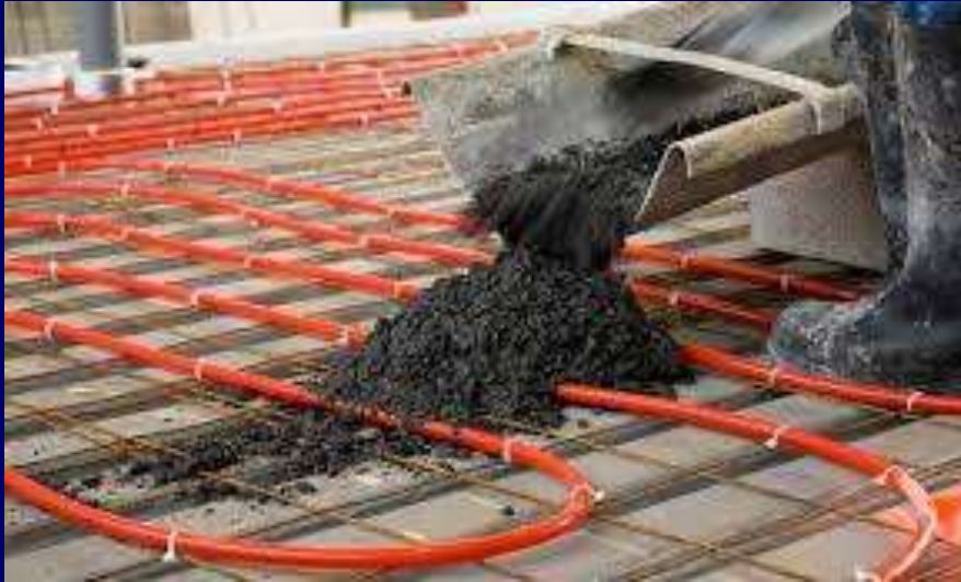
Electric Heating Wires
